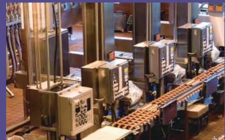
Distributed Monitoring and Control Systems
